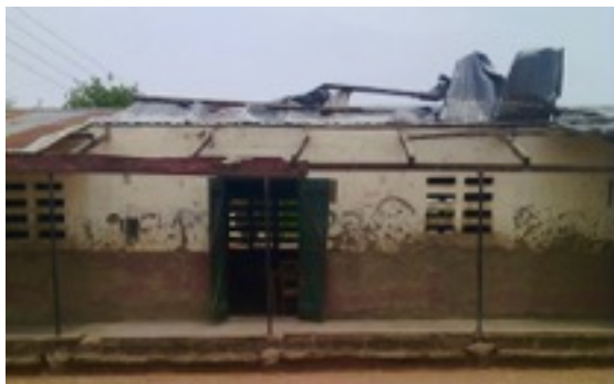
Kubori - in Dilapidated Condition
